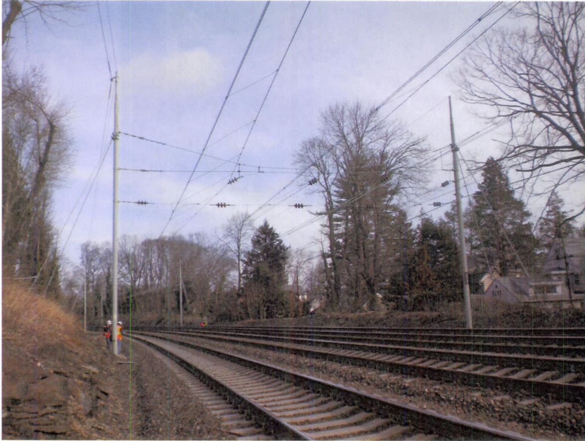
Figure 3 - Existing Catenary Structures
