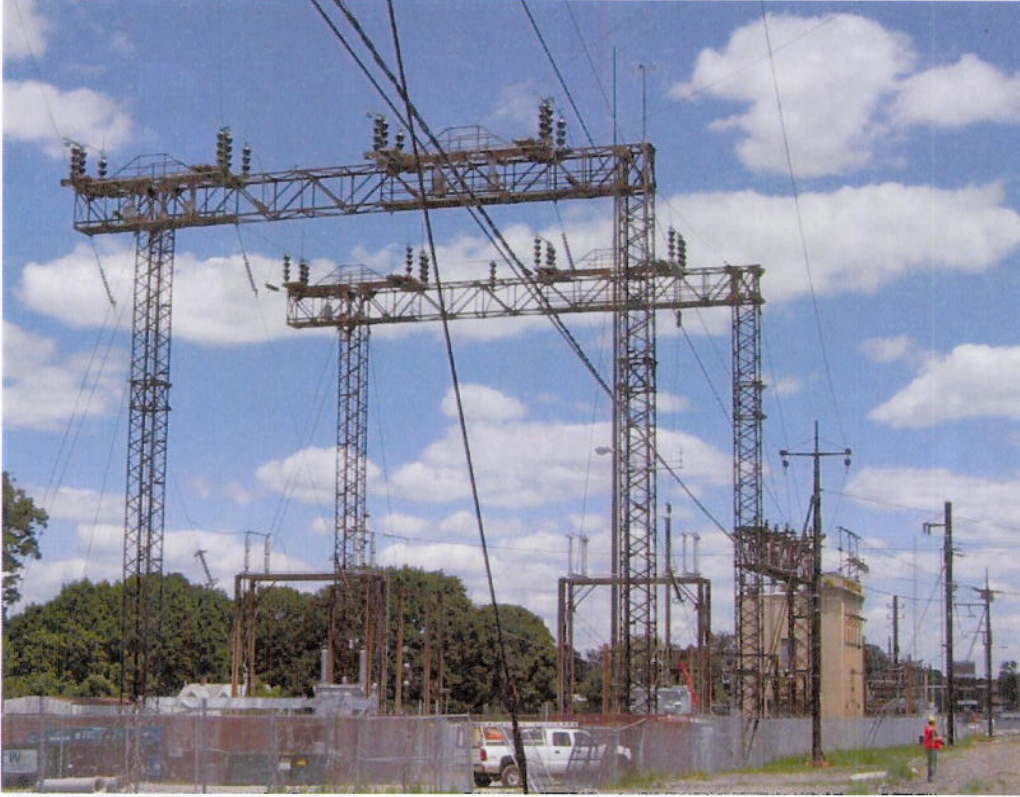
Figure 6 - Paoli Substation, 138 kV Structures
