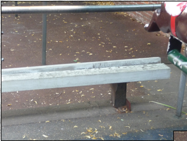
Benches in Need of Repair
