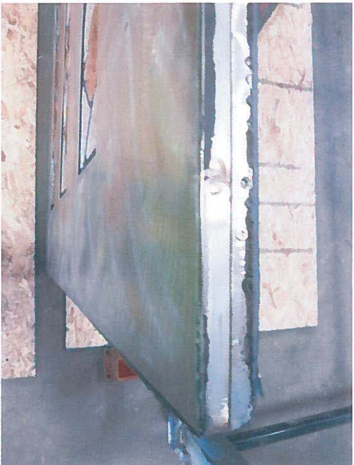
Edge of the panel with deteriorated sealant
