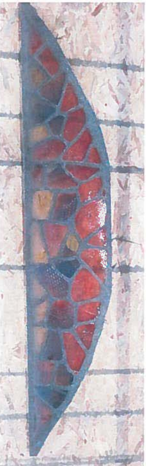
Fanlight – note the discoloration due to soiling at the base
