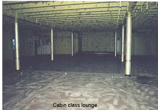
All of her interiors are now completely gutted.
