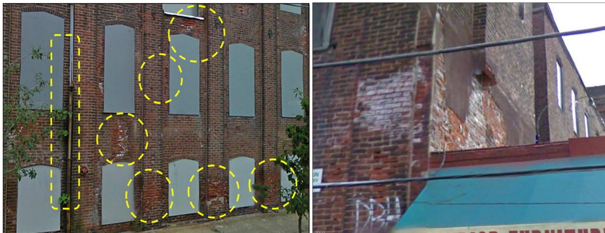
Structural defects along Boston Street, adjacent to showroom (NIOSH)
